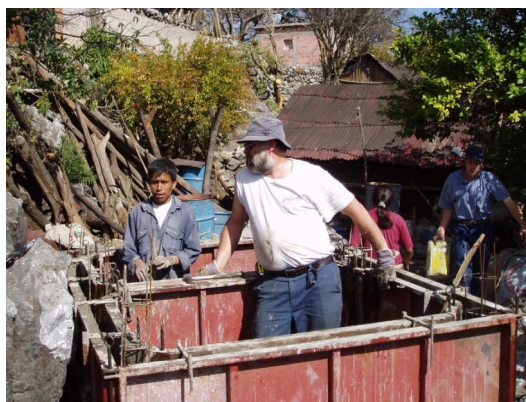
David & Diacono, a local constructor, installing the mold prior to pouring toilet vaults.
